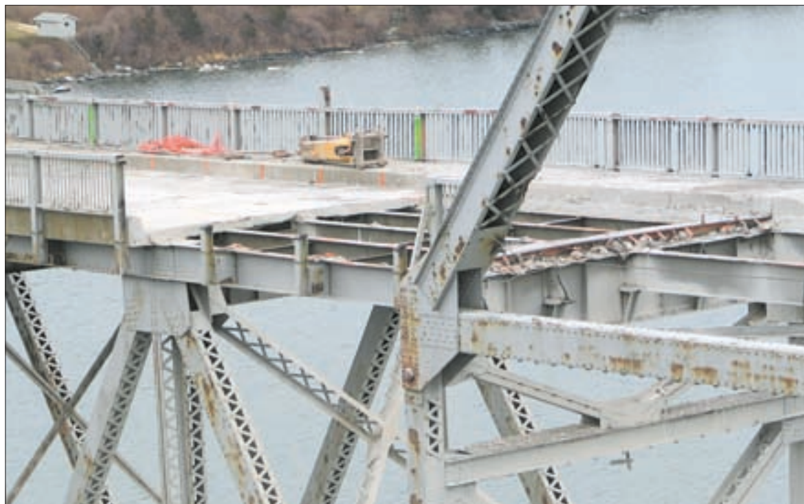
Workers have been removing the decking from the old Jamestown Bridge in preparation for blasting the superstructure. Photo by Joe Logan
