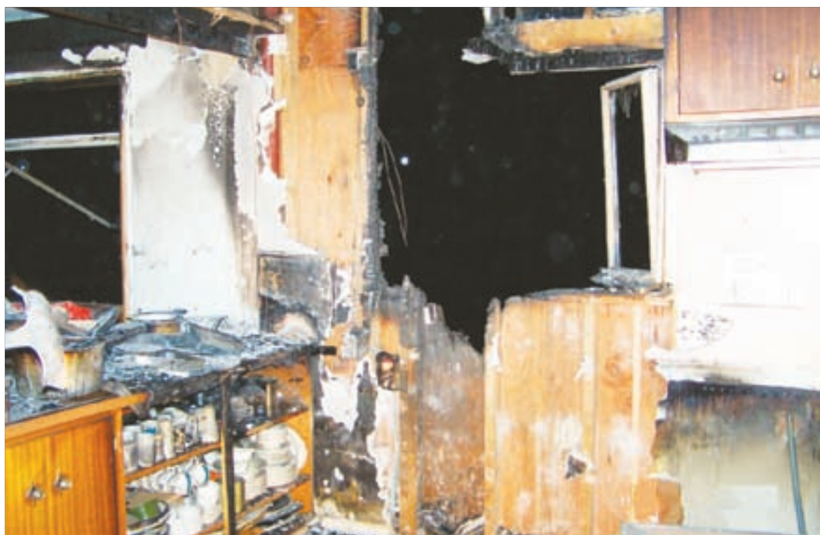
The fire started in the kitchen at 265 Highland Drive. Photo courtesy Jamestown Fire Department
