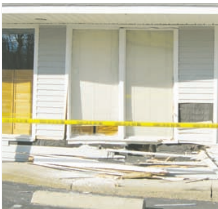
Doctor's office damaged by car Damage to Jamestown Family Practice on Southwest Avenue was extensive after a car drove into it. See story page 3. Photo by Jeff McDonough
