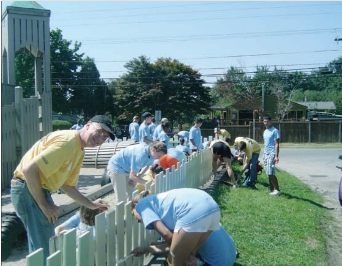
Almost 200 Providence College freshmen visited Jamestown last Saturday for a day of community service. Here, volunteers paint the fence at the community playground.
